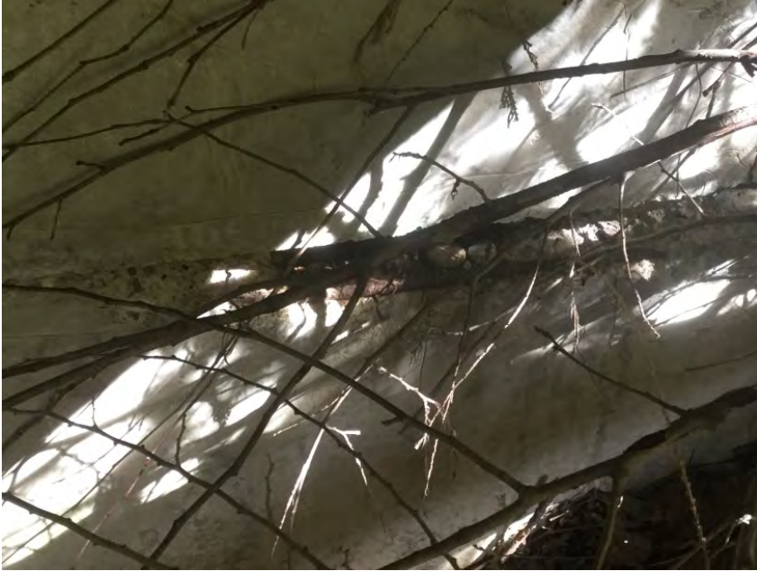
Right bank fill retainment structure damage
